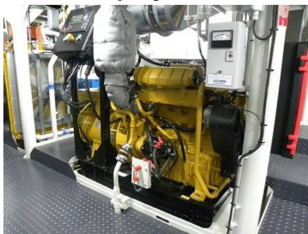
Caterpillar generator set
