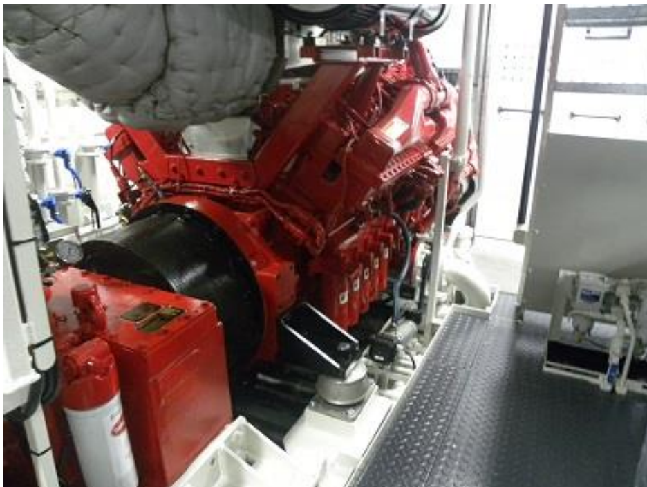
Starboard side Main engine
