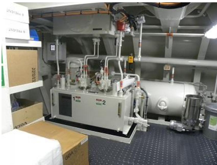
Hydraulic power pack
