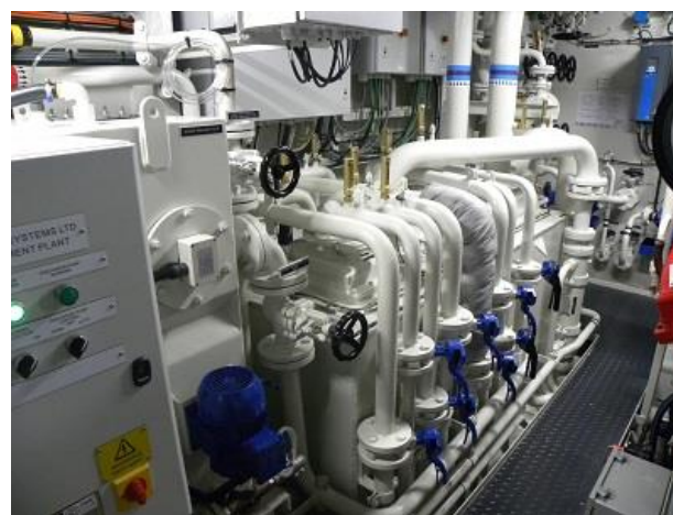
Starboard side Box cooler
