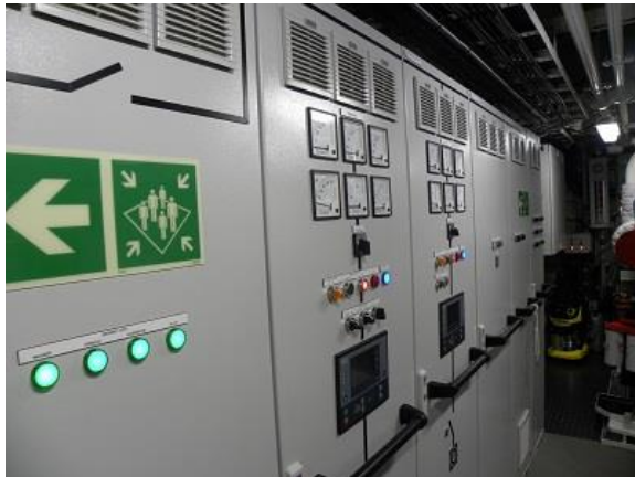
Main switchboard Portside view
