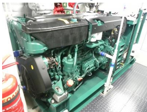
Starboard side Volvo generator set
