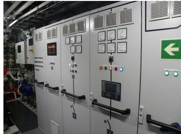
Main switchboard Starboard view
