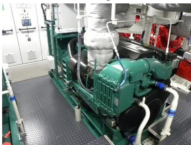
Portside Volvo generator set
